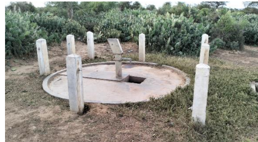
An abandoned, broken water point. The project will repair such infrastructure and maintain it for years - financed by user fees and revenues from the sale of carbon credits.
